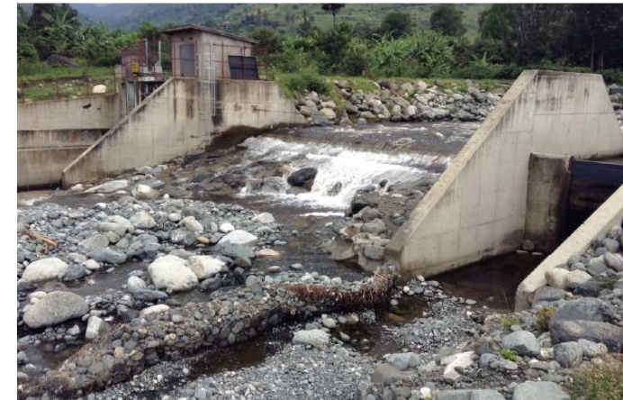
Bugoye Hydro Project - Uganda - 13 MW Final Investment Committee
