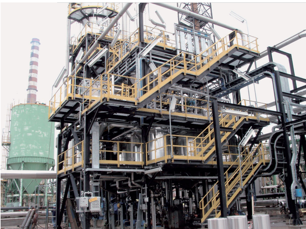
LIFE demonstrates the relevance of emerging or insufficiently developed techniques. The picture shows the new regeneration unit of the Sanazzaro refinery (p. 22).
