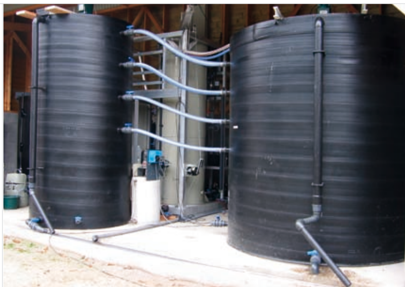
ZNP's prototype facility for treating livestock manure
