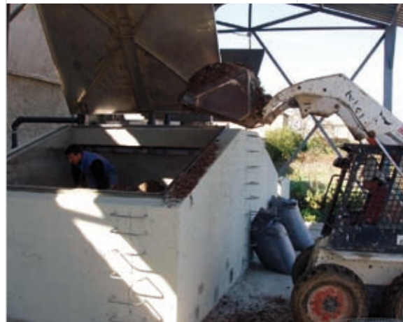
Project results provide alternative uses for fermented grapes and offer useful waste minimisation benefits
