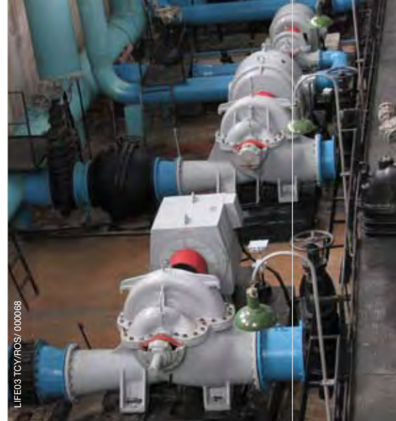
Some units of Kaliningrad's large water and heating supply companies participated at the MEEMAS project
