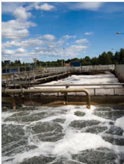
The open air bioreactors contain thousands of plastic Biofilm carriers
