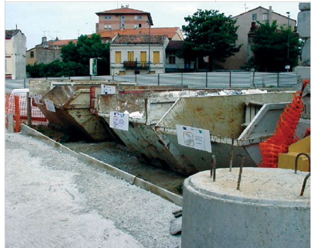
Large containers facilitate sorting of special waste such as timber, window grates, cables and iron.
