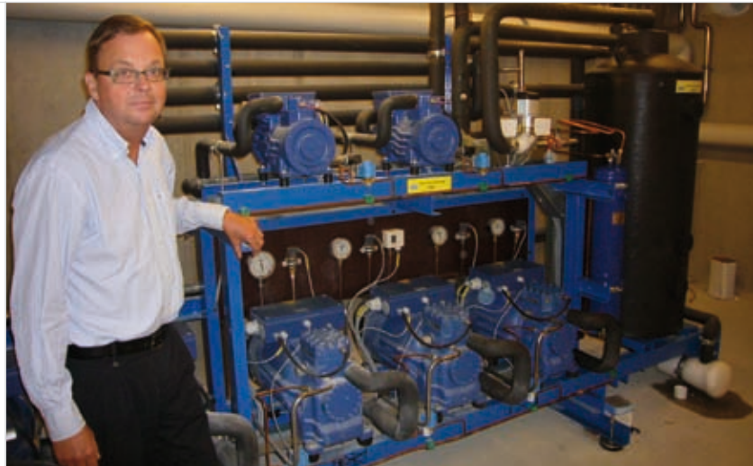
Finn Christensen presents the CO 2 Ref compressor system installed in a Roskilde supermarket
