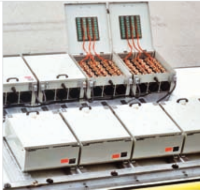
Close-up of ultracapacitors.
