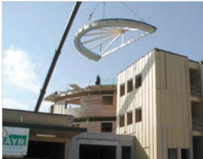
The prefabricated building's wooden structure and its cladding were assembled in just nine days.
