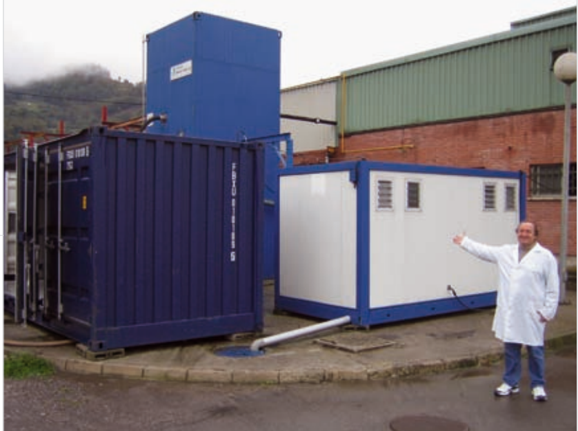
A horizontal transport container houses the hydrolysis tank, the heating system, the control panel, two pumps and a macerator.
