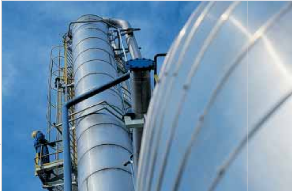
Better management of industrial risks is one of the most important advantages of environmental management systems: Distillation towers at Speichim Processing, Plaine de l'Ain industrial estate, France.
