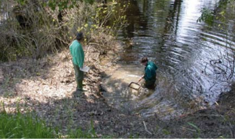
The project secured a water supply to dry areas by excavating the channels of the flood plain
