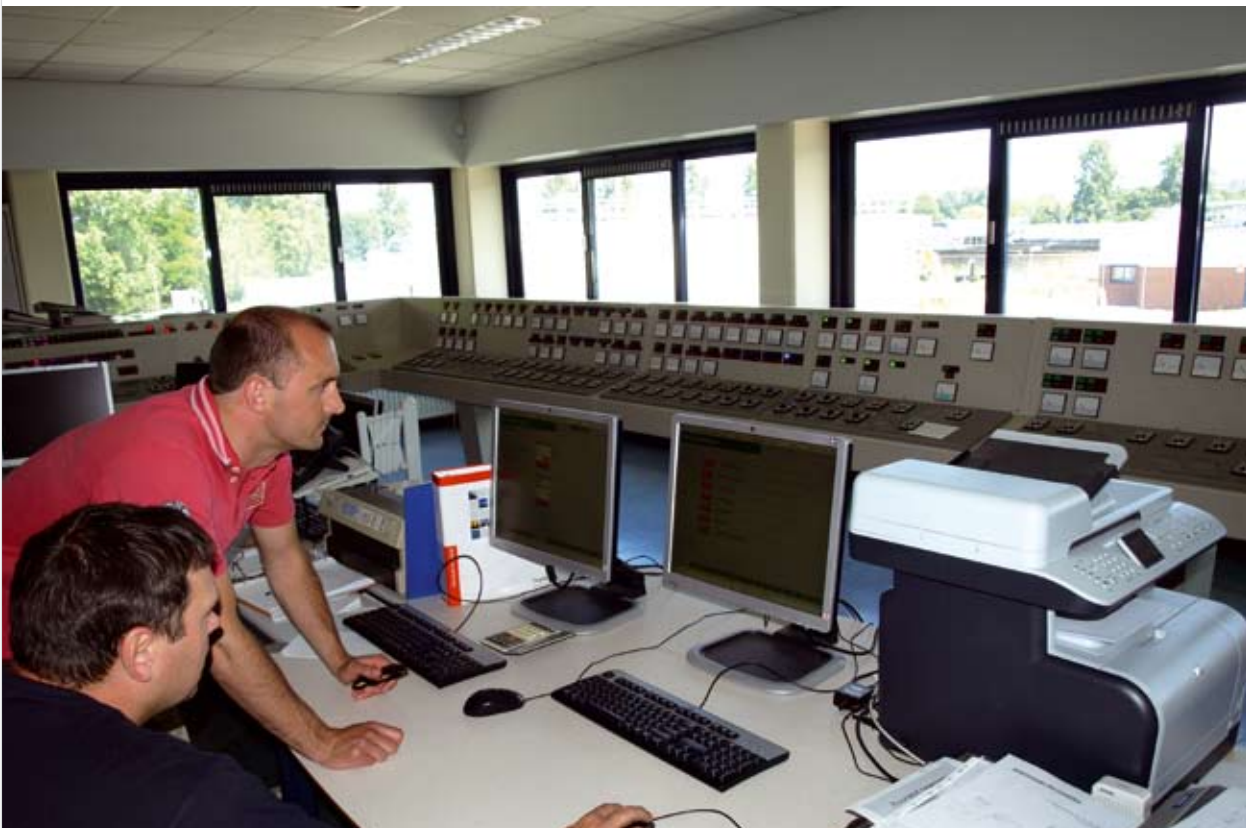
The continuous sand filter is monitored from this control room
