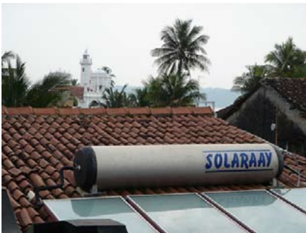
© M. Renner, 2005 Solar thermal panels on the Ocean View Guesthouse. Sri Lanka.
